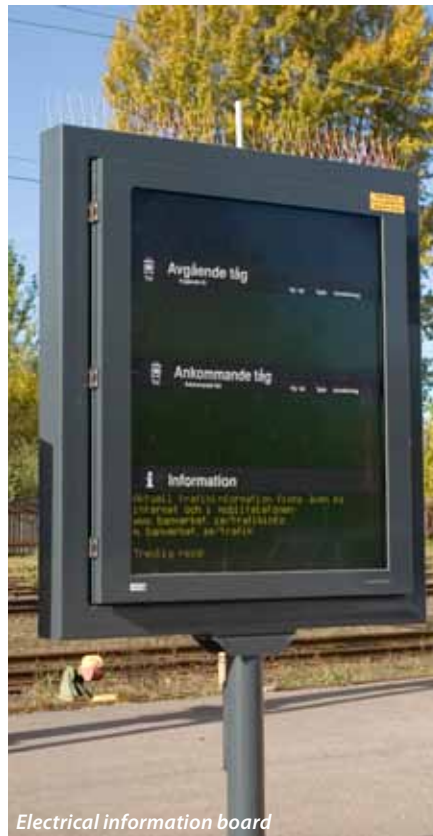
Electrical information board
